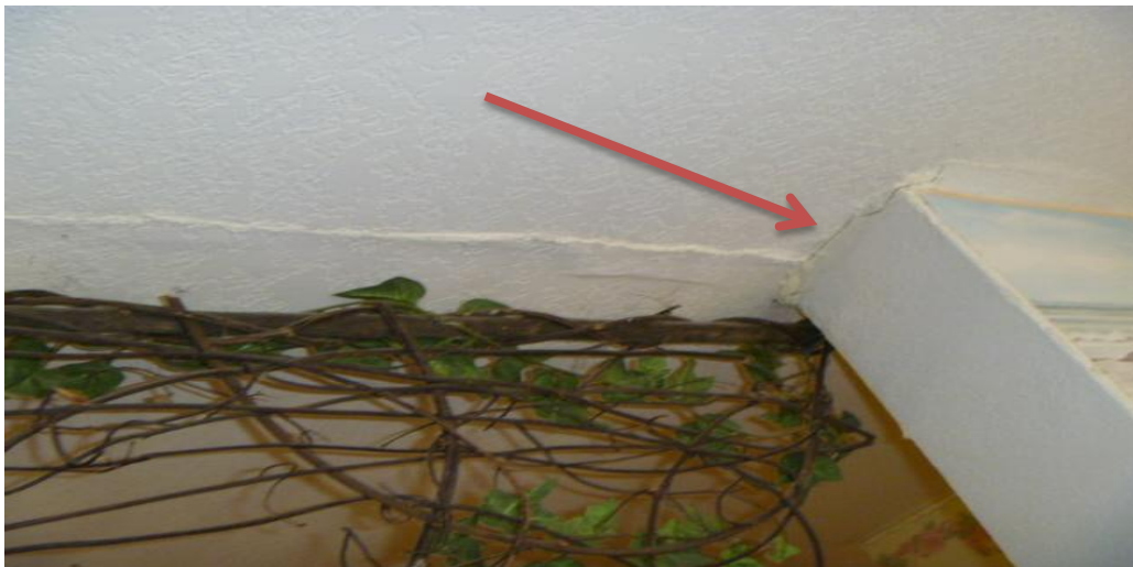
Figure 9 Truss uplift cracks
