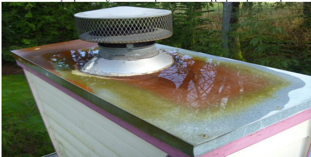
Figure 4 Rust on chimney cap
