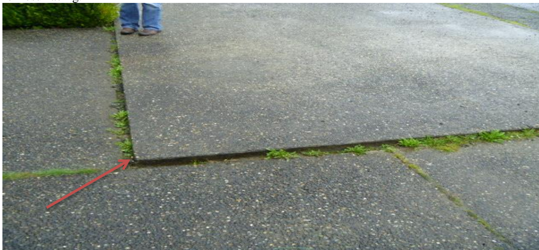
Figure 5 Resurfacing of driveway needed
